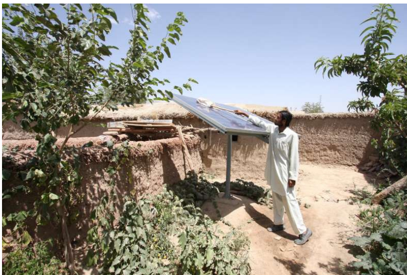
A resident of Ferozai Kan village in Balochistan, Pakistan tends to two solar panels which power the area's water supply. © UNHCR/T.Irwin
